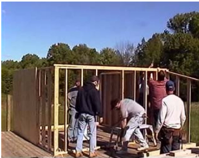
In April 2006, construction of a new building begins. It is to house the newly acquired 12" Meade reflector from Lakeview High School. It was a donation late in 2005.
